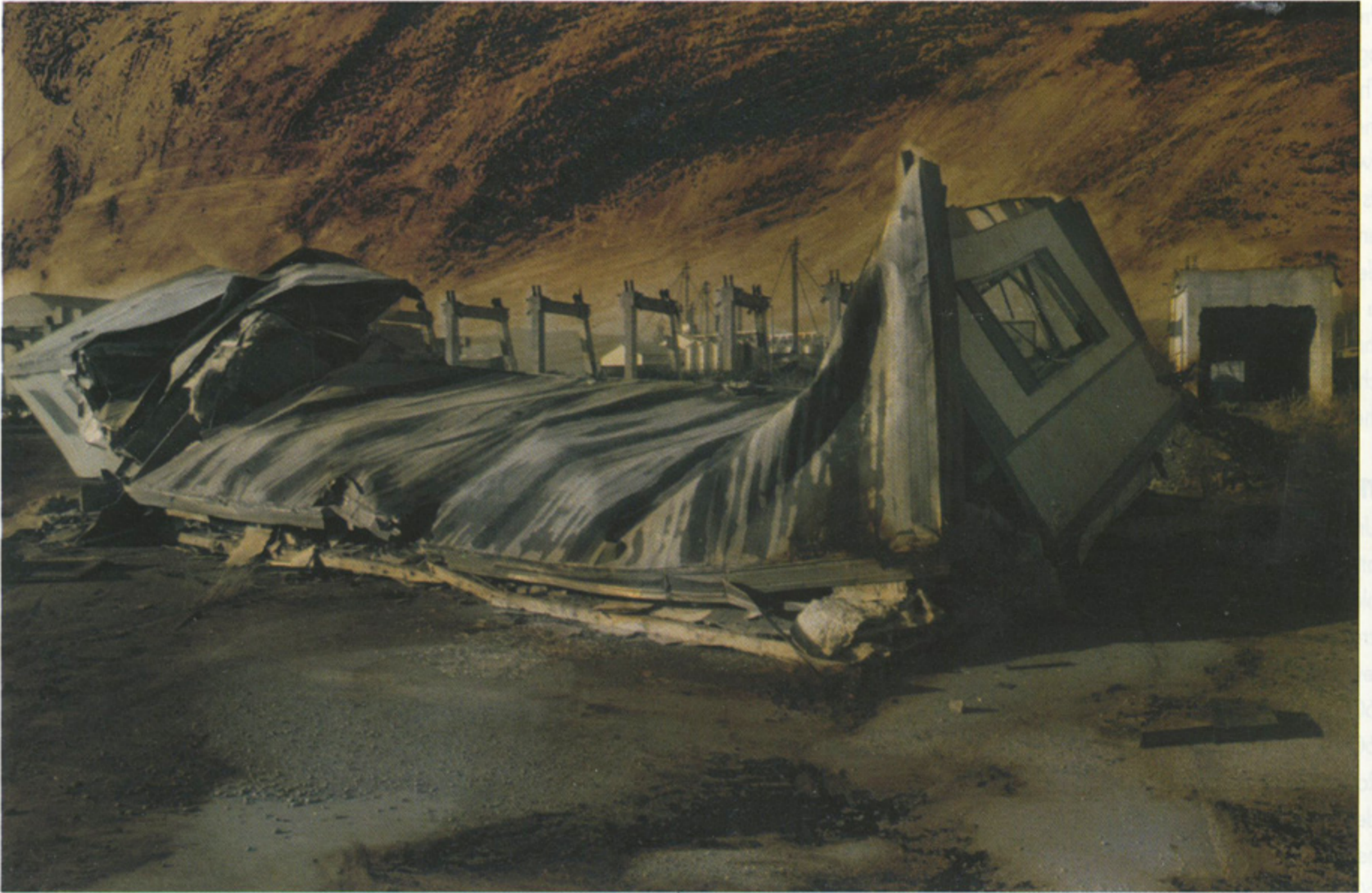
Collapsing Shelter, Tillamook, Oregon Air Force Base, 1996
